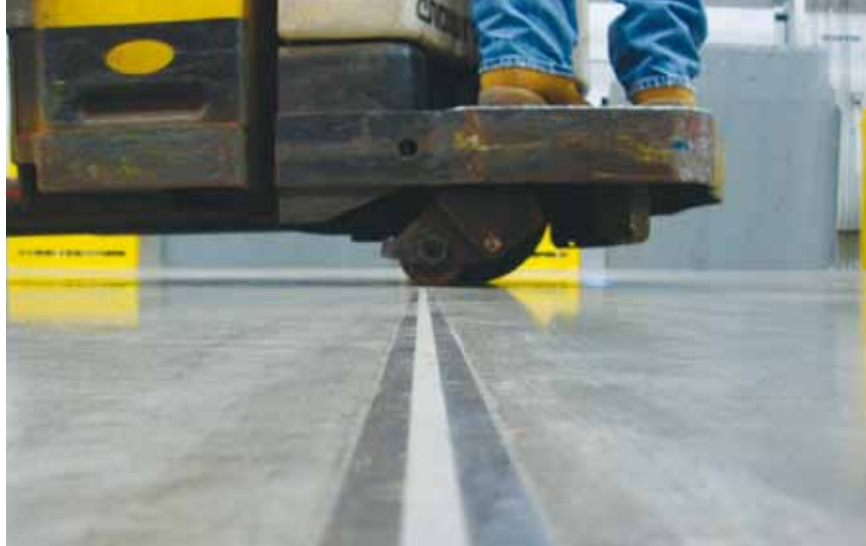
Properly designed and constructed joints are critical to achieving a durable floor. PHOTO: MIKE HAAG
