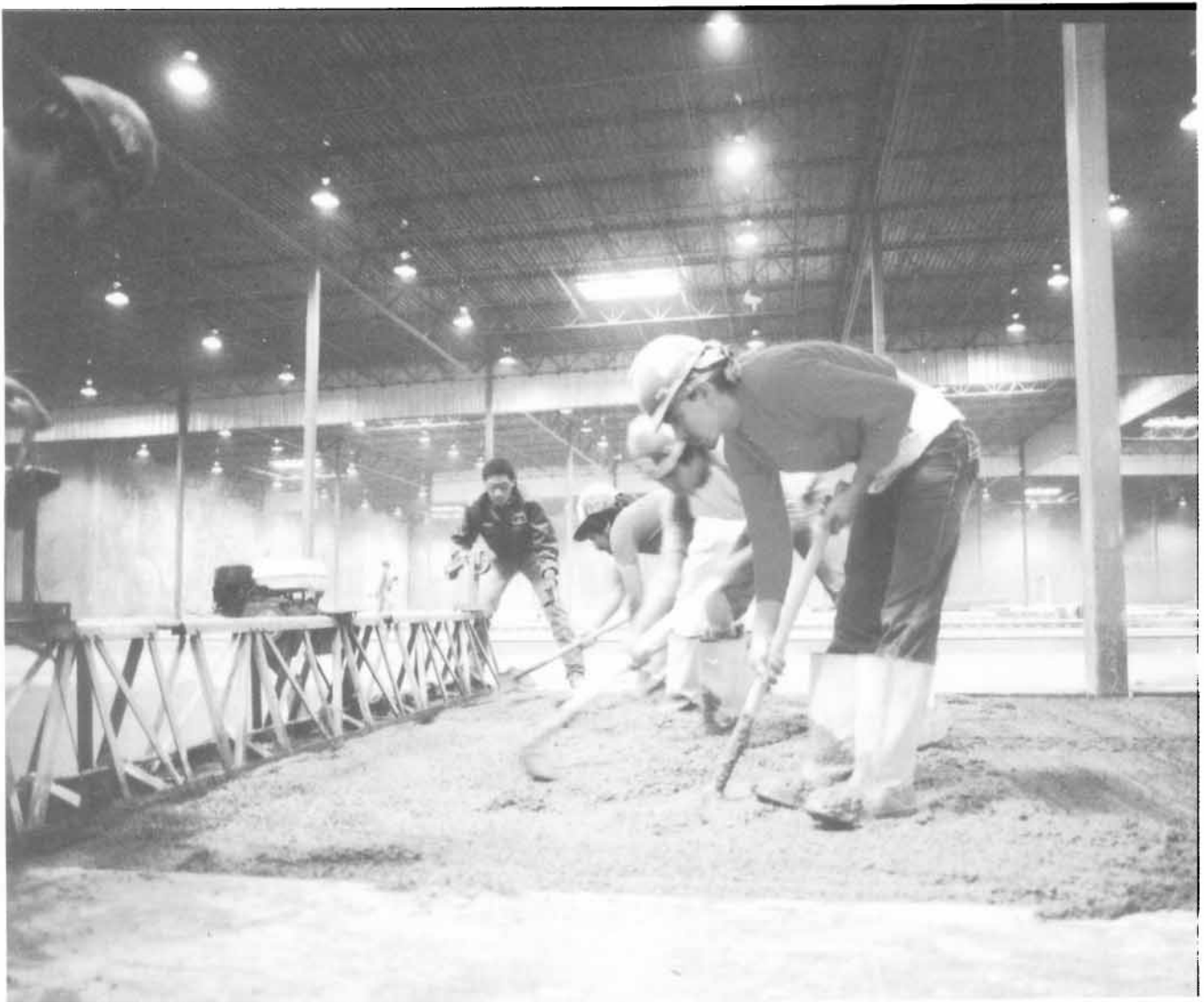
Competing against themselves, the flooring crew worked to create section after section that far exceeded an F100 rating.
